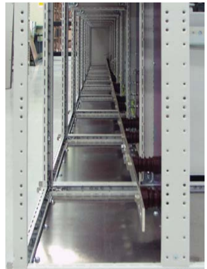
Generous space in the rear of the cabinet makes cabling your soft starter easy. The MVS has options to cable from either bottom, top, left or right.
