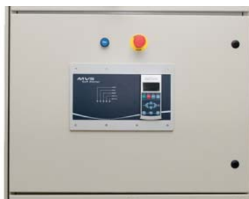
Lockable door prevents unauthorised access.
