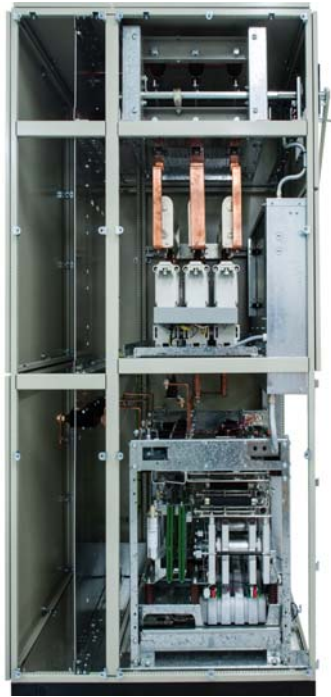
Side view of MVS panel with panels removed.
