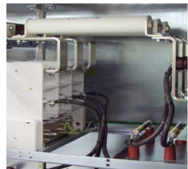
Contactor and fuse detail.
