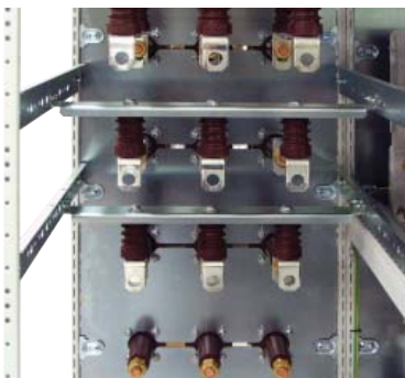
Transition panels may be cabled into or use busbars.
